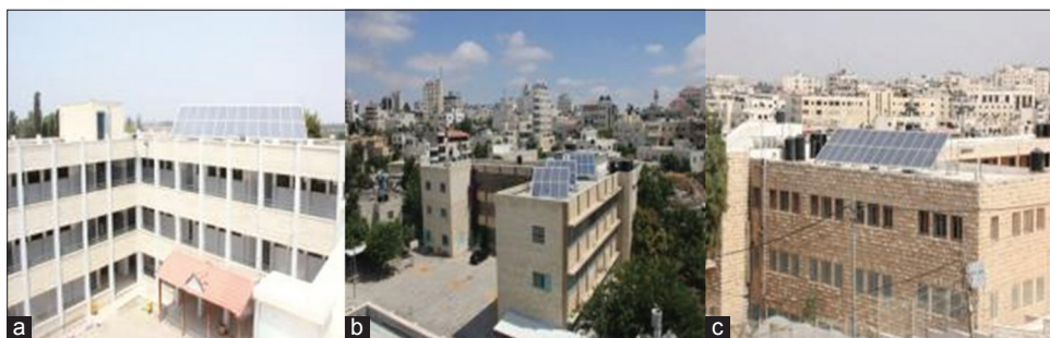
Figure 7: Grid-connected power plants – (a) Alrazi, (b) Khawla Bent ALazwar, (c) Alumeh school
